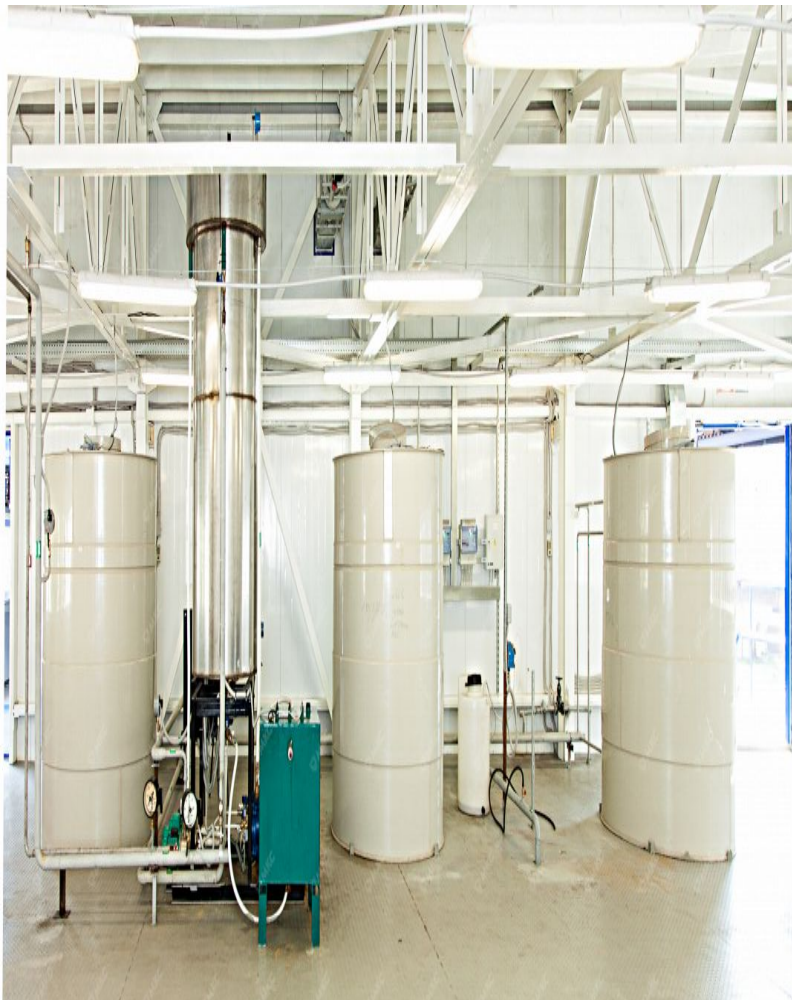
The trigeneration system implemented at the facility of the MKS Group
