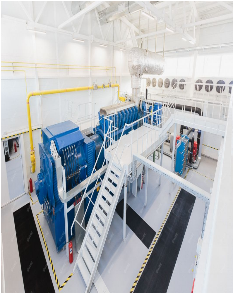
Cogeneration plant (CHP) at the facility of the MKS Group
