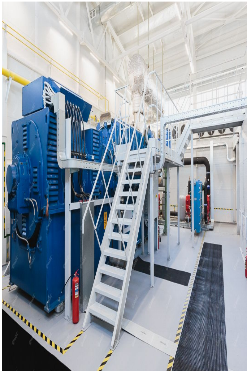
Cogeneration plant (CHP)
