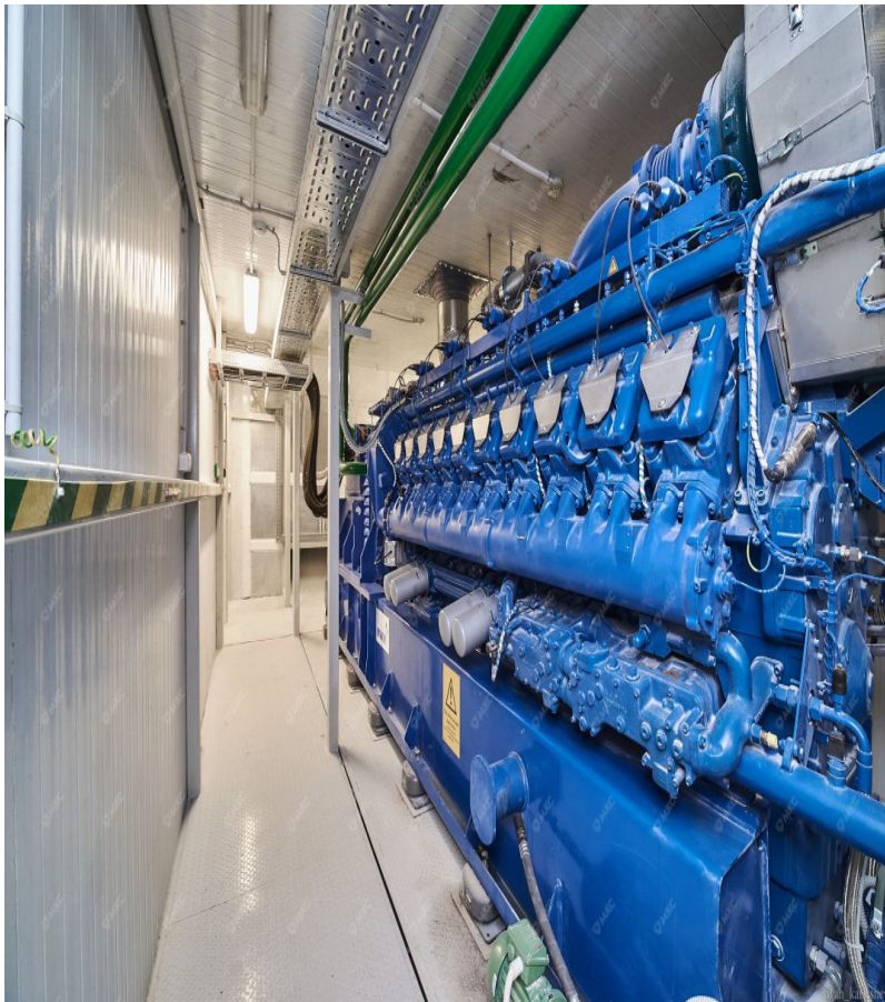
Cogeneration plant (CHP) at the facility of the MKS Group
