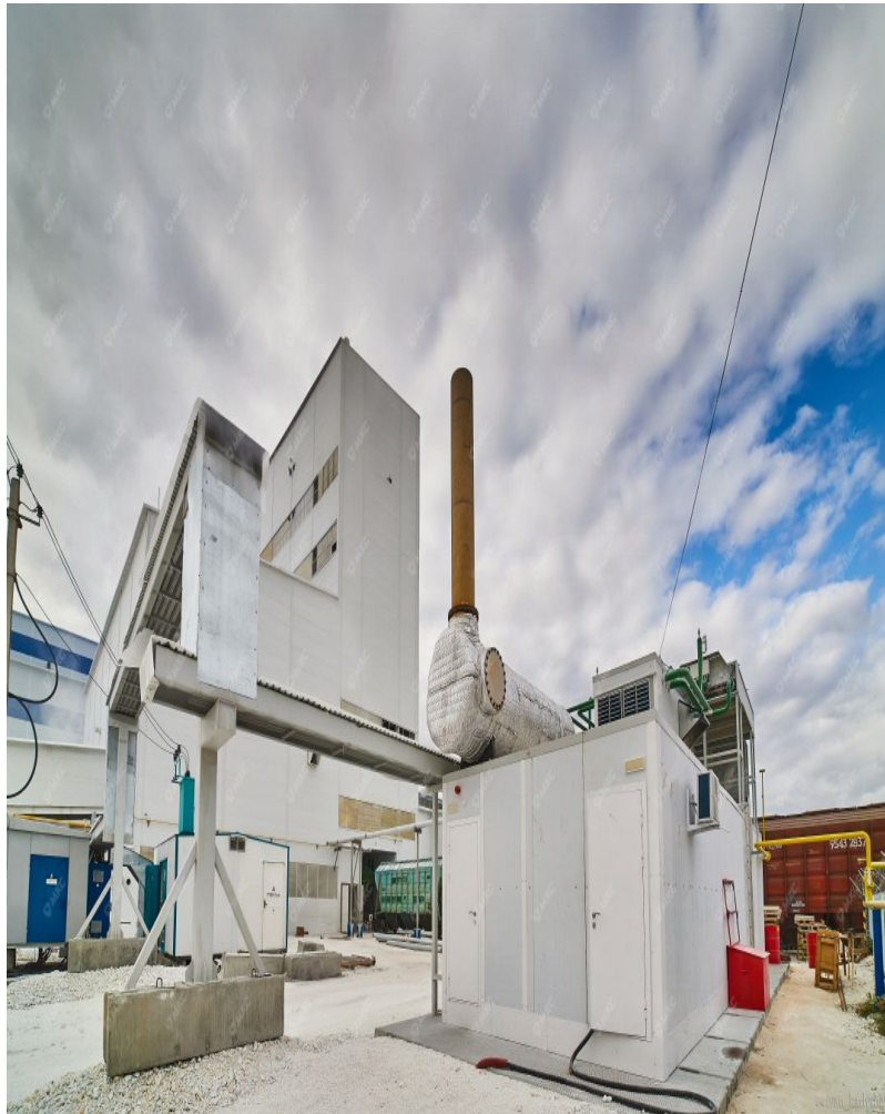
CHP-plant produced by the MKS Group as part of the enterprise for the extraction and processing of natural stone
