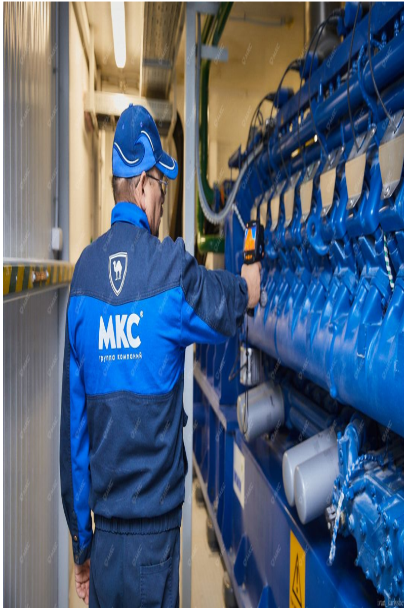
Cogeneration plant (CHP) at the facility
