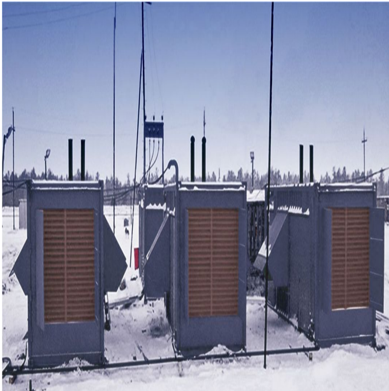
photos of energy complexes based on diesel power plants
