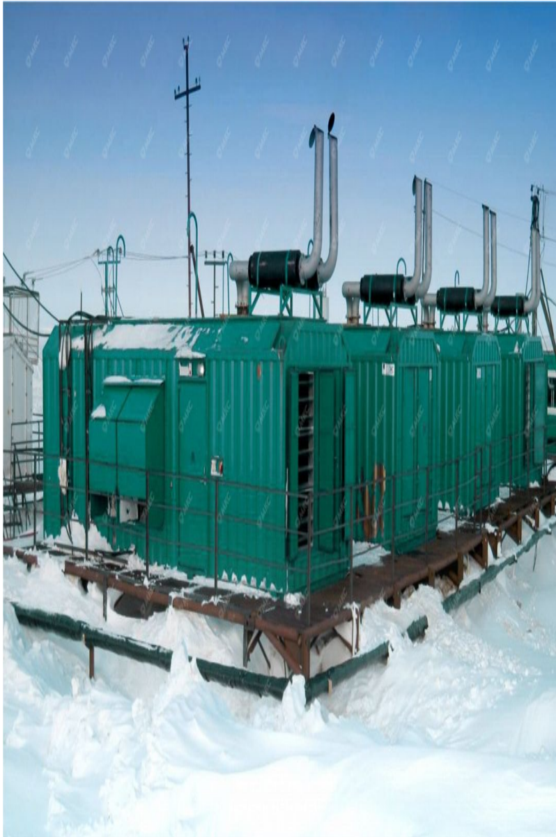
photo of diesel power plant
