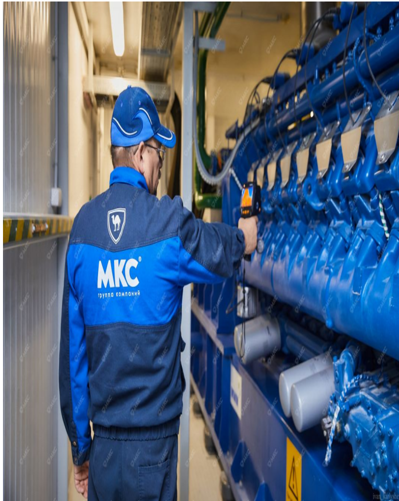
MKS Group employee measures the temperature of the MWM engine exhaust gas line using a thermal imager
