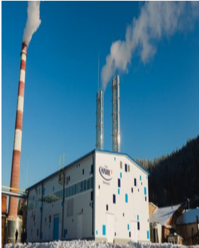
photo of a stationary version of a gas piston power plant
