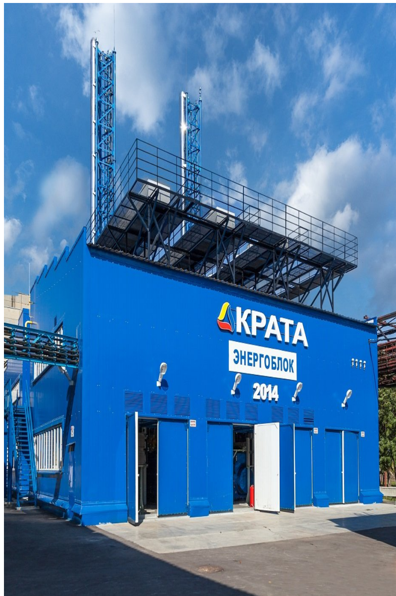
Trigeneration power center of the chemical products plant of Pigment JSC
