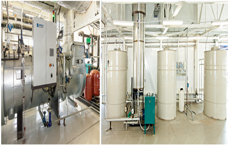
Trigeneration system implemented at MKS Group's facility
