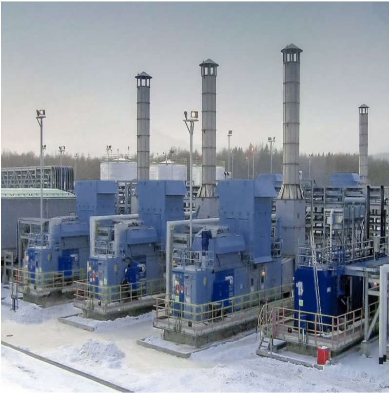
Stationary gas-turbine power plant
