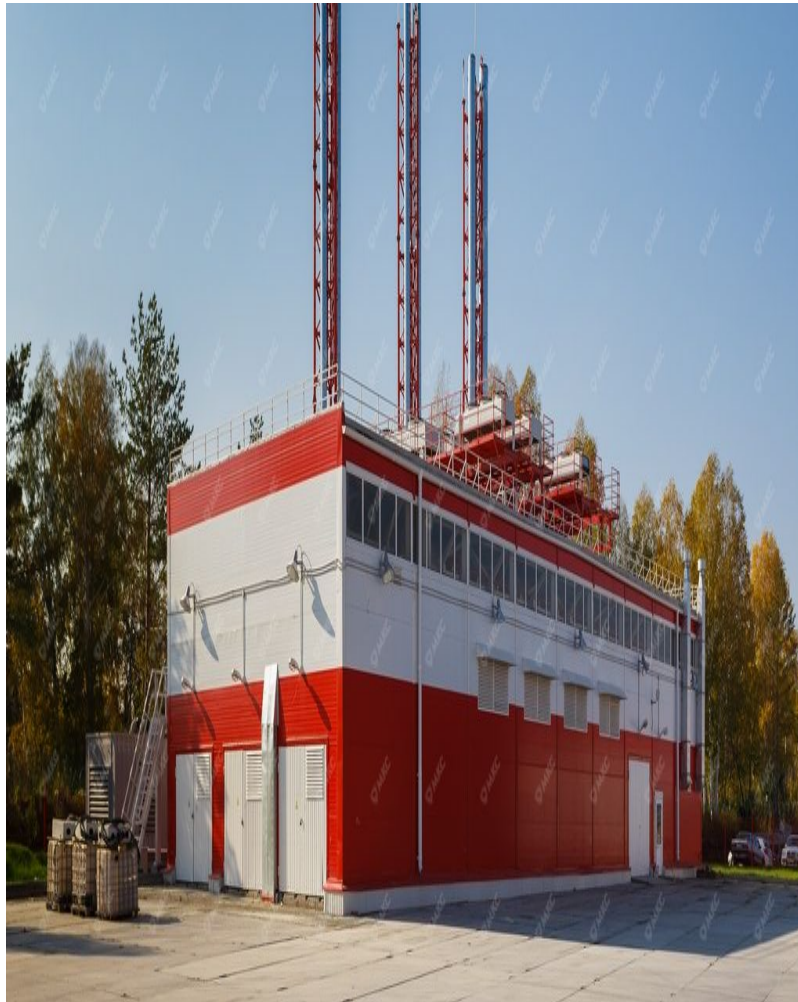
an example of a stationary power plant produced by the ISS Group of Companies
