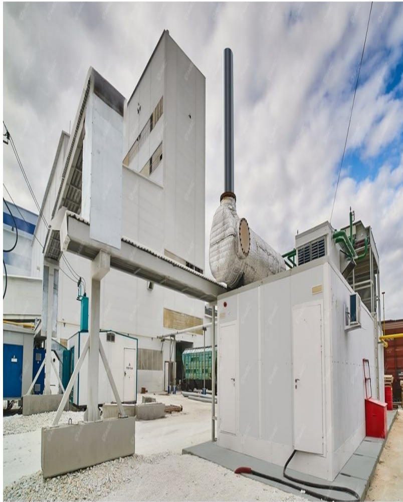
own electricity generation for the enterprise
